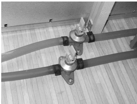
Fig. 100: Drain valves opened
