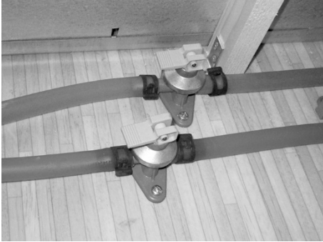
Fig. 151: Closed drain valves
