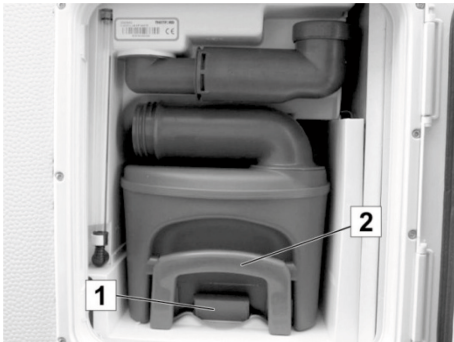
Fig. 172: Waste holding tank in the disposal shaft
