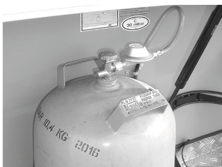
Fig. 77: Gas bottle with low pressure regulator and low pressure hose
